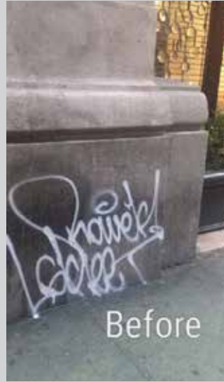
Vandalism in front of our station (before).
